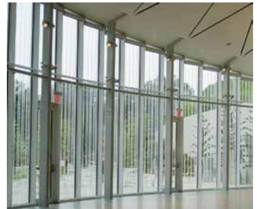
Glass walls and doors at the Brooklyn Botanic Garden's Visitors Center include a custom fritting pattern that meets bird-friendly criteria. Monitoring for collisions after the building opened indicates that the design was successful. Photo by Christine Sheppard, ABC
